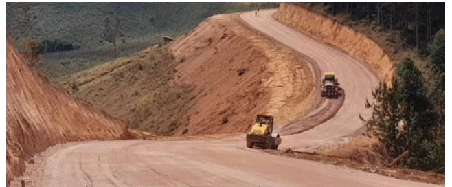
Compacting the base surface after the soil has been mixed with Ecoroads solution at Mufindi- Sawala- Lulanda Road, Mufindi
