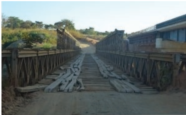
Nampungu Bridge on the Tunduru – Matemanga Road, June 2016. To the right, a new bridge is under construction but was not mentioned by the couple who took the photo!
