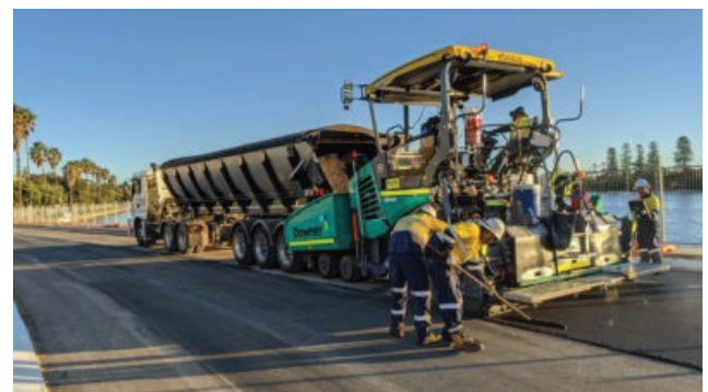
Asphalt with the additive TonerPlas, made from mixed soft plastics, is used to resurface a roadway in Fremantle, Western Australia
