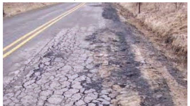
A road section in failure mode
