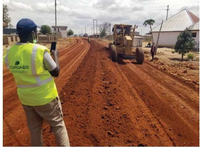
Mixing soil with Ecoroads solution to obtain a uniform soil mixture with optimum moisture content at Chamwino, Dodoma
