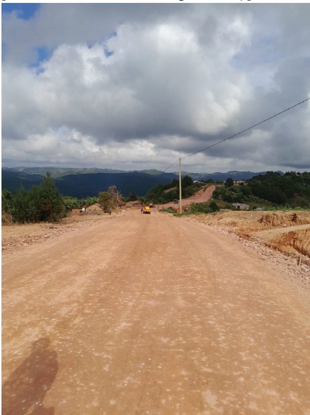
Compacting the base surface after the soil has been mixed with Ecoroads solution at Mufindi- Sawala- Lulanda Road, Mufindi
